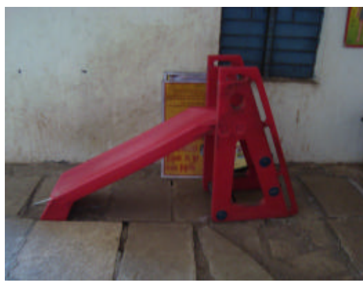
Broken flooring on which the slide is placed
