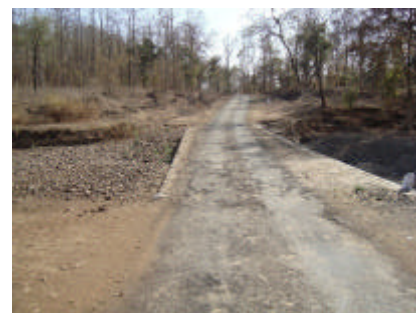
Bridge that gets flooded during monsoons
